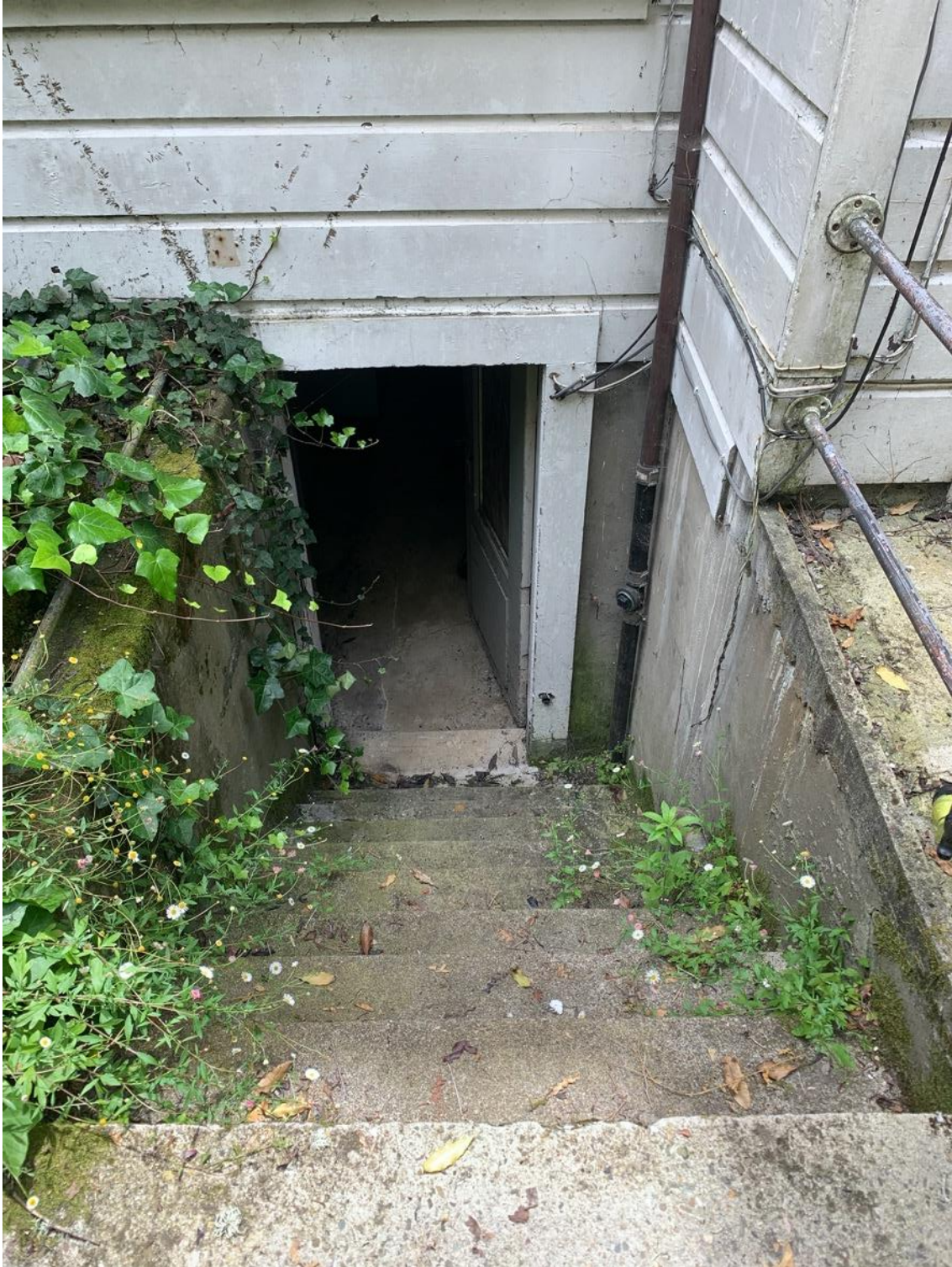
3312-14 Clay Street. Detail View of Steps to Basement and Rear Basement Door. North-Facing Rear Elevation, Looking South
